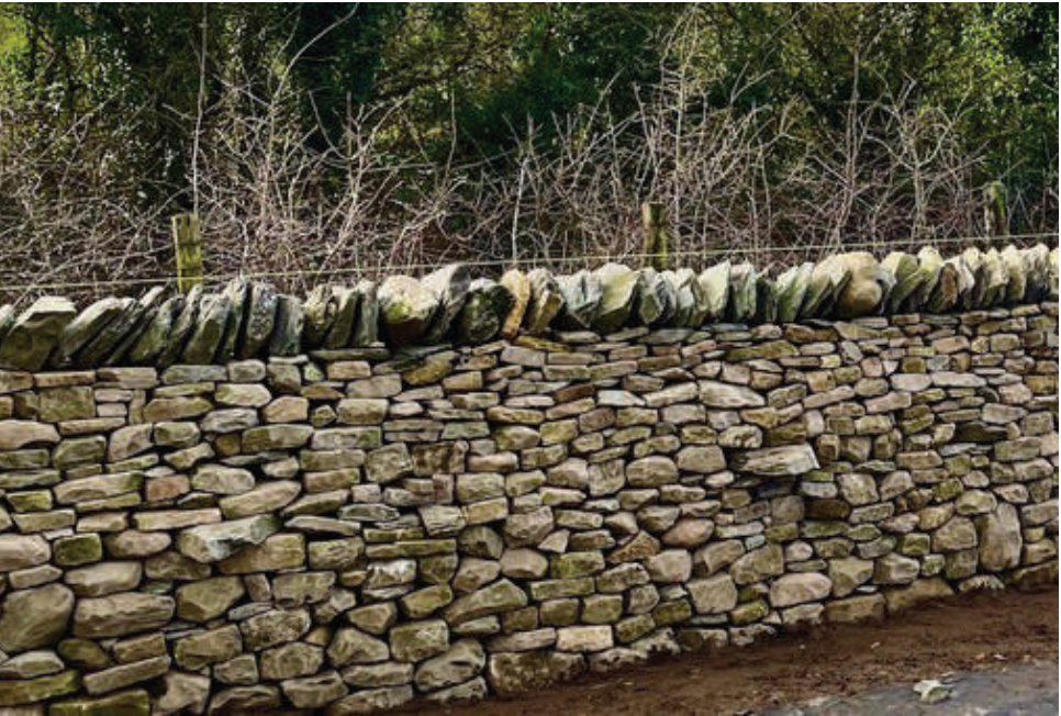
4. This wall is incomplete - where is its dressing ?
